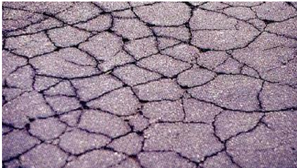
Fig. 1. Fatigue cracks in asphalt pavement
